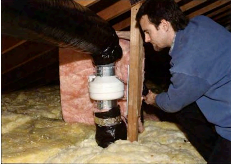
In-line Exhaust Fan Ventilation ( Click to Return to Section )
