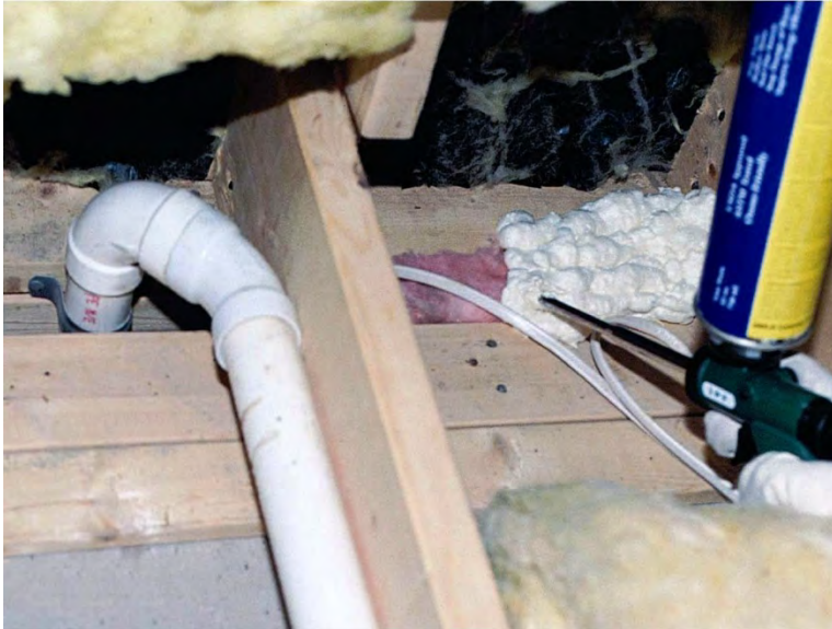
Plumbing Wet Wall Sealed with Fiberglass Batt Backer and 1-Part Foam ( Click to Return to Section )
