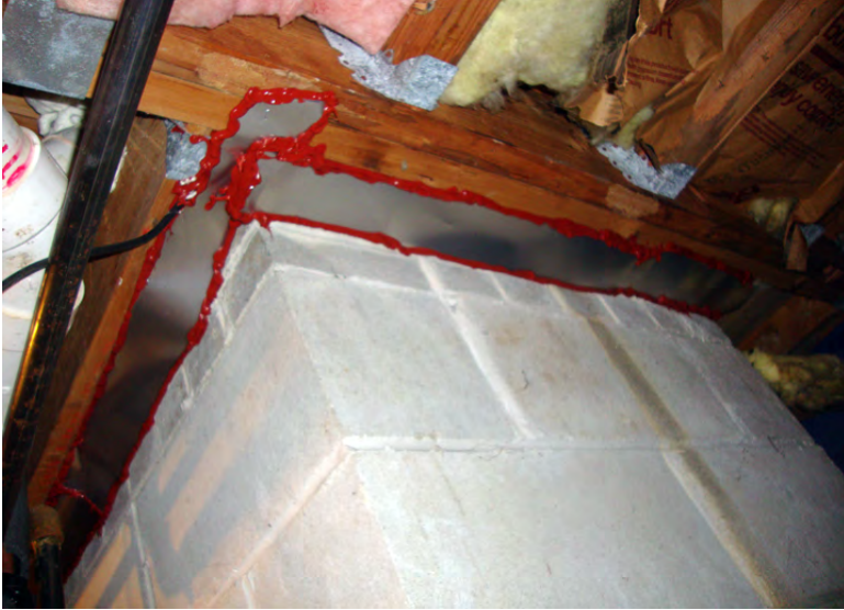
Chimney in Basement Sealed with Sheet Metal and High-Temp Caulk ( Click to Return to Section )
