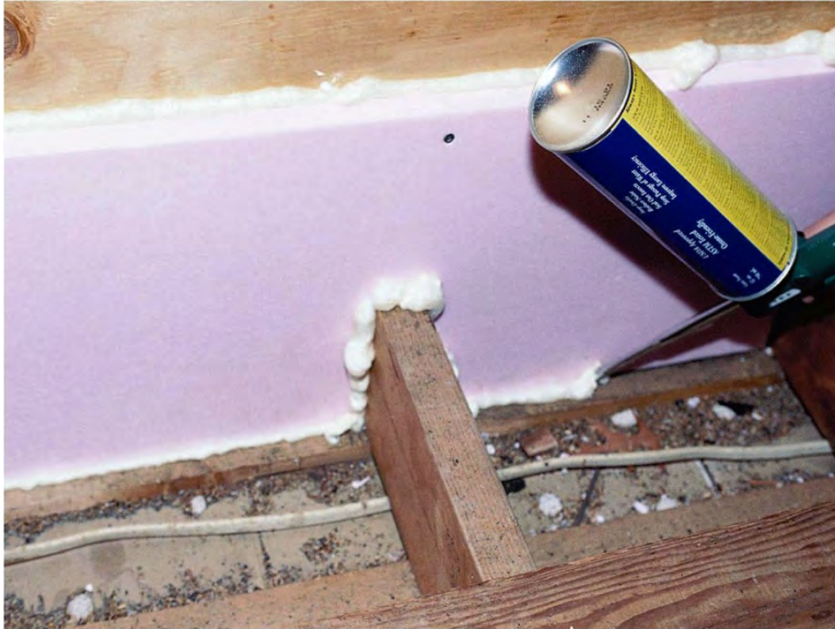
Knee Wall Transition Sealed with XPS and 1-Part Foam ( Click to Return to Section )
