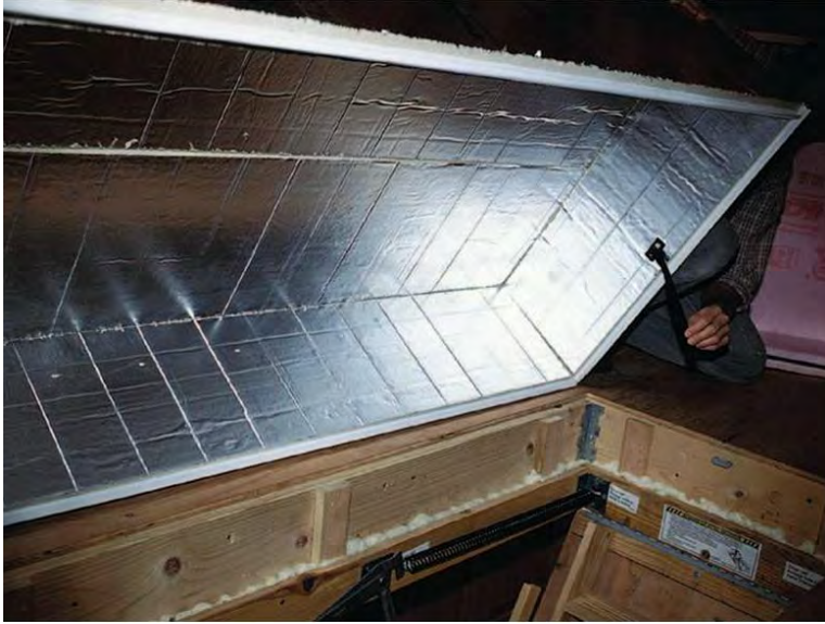
Pull Down Staircase Enclosure ( Click to Return to Section )
