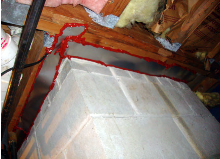
Chimney in Basement Sealed with Sheet Metal and High-Temp Caulk ( Click to Return to Section )
