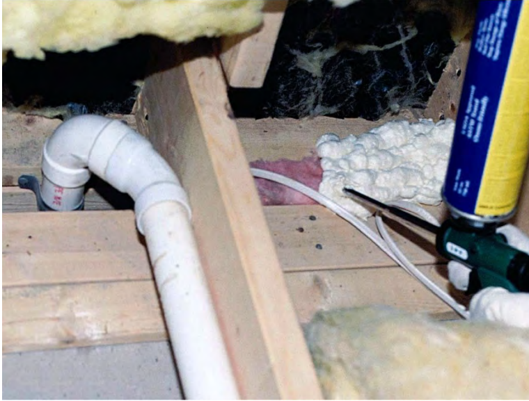
Plumbing Wet Wall Sealed with Fiberglass Batt Backer and 1-Part Foam ( Click to Return to Section )
