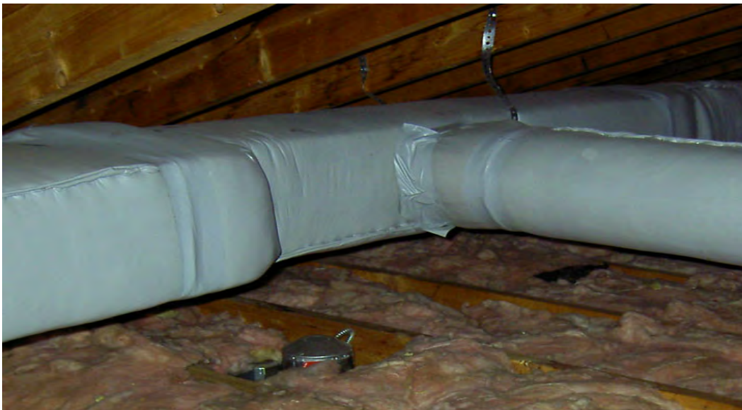
Sealed Vapor Retarder on Attic Ductwork ( Click to Return to Section )
