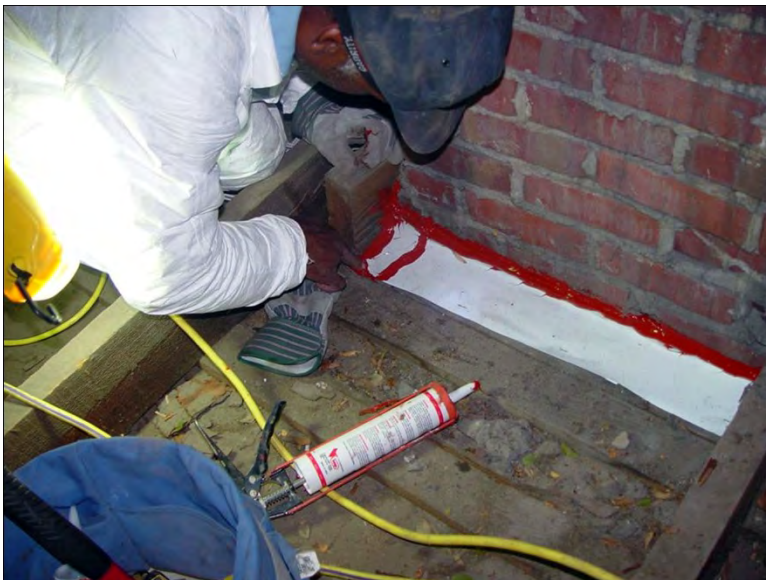
Chimney in Attic Sealed with High-Temp Caulk and Metal Flashing ( Click to Return to Section )
