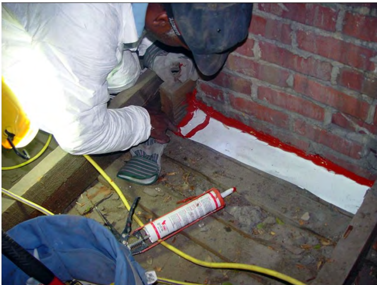
Chimney in Attic Sealed with High-Temp Caulk and Metal Flashing ( Click to Return to Section )
