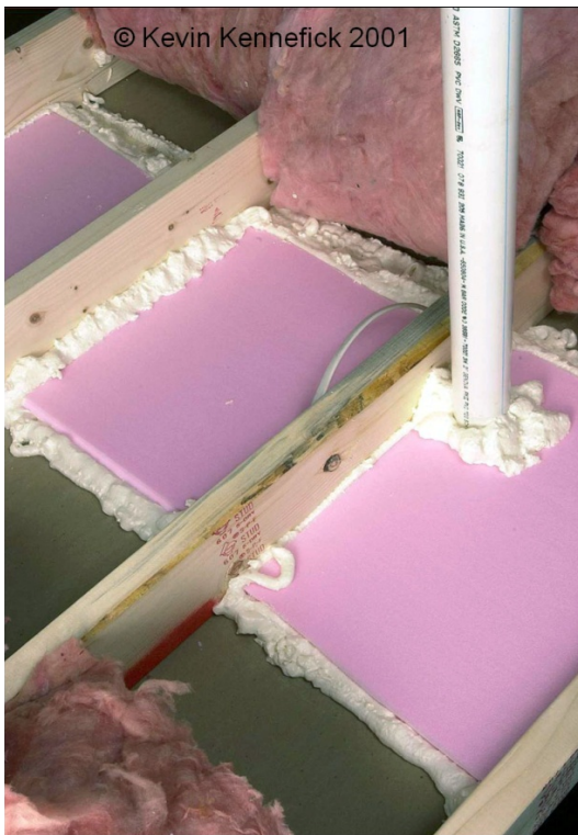
Dropped Soffit Sealed with XPS and 1-Part Foam ( Click to Return to Section )
