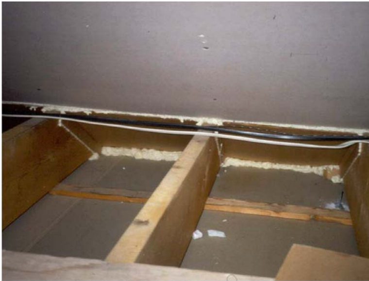
Kneewall Attic Air Sealed Along Rafter Line (attic space within thermal/pressure boundary) ( Click to Return to Section )
