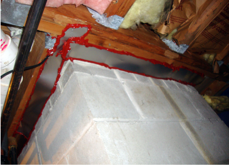
Chimney in Basement Sealed with Sheet Metal and High-Temp Caulk ( Click to Return to Section )
