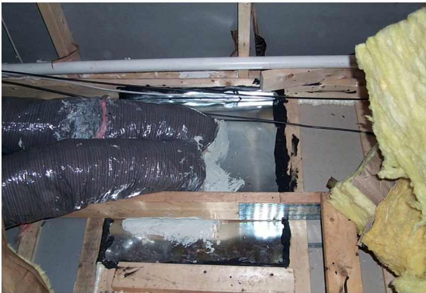
Open Attic Chase Sealed with Sheet Metal, Duct Mastic and Acoustical Sealant ( Click to Return to Section )
