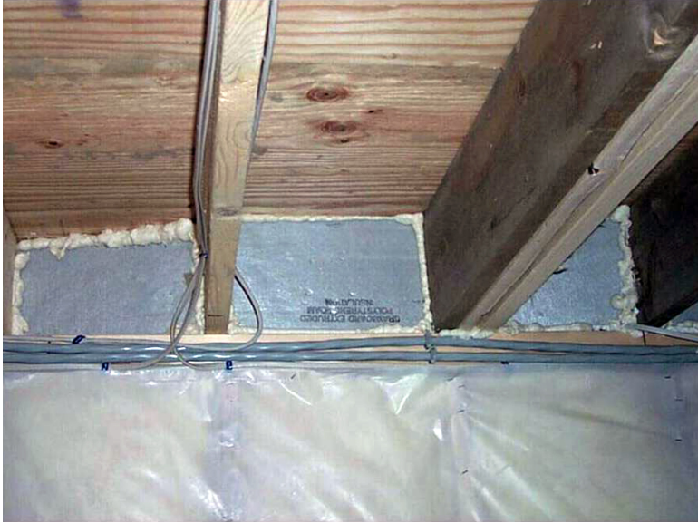
Rim Joist Insulated (and Sealed to Sill) with Foam Board and 1-Part Foam ( Click to Return to Section )
