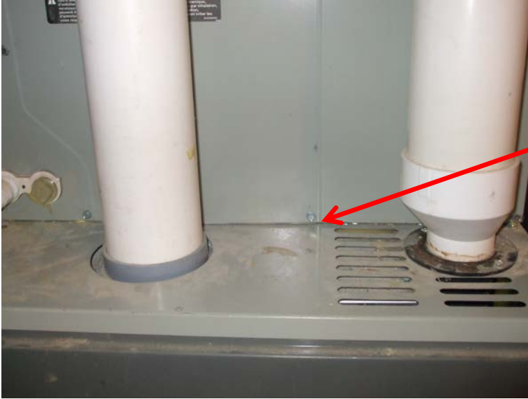
Air Handler Sealed with Silicone Caulk ( Click to Return to Section )
