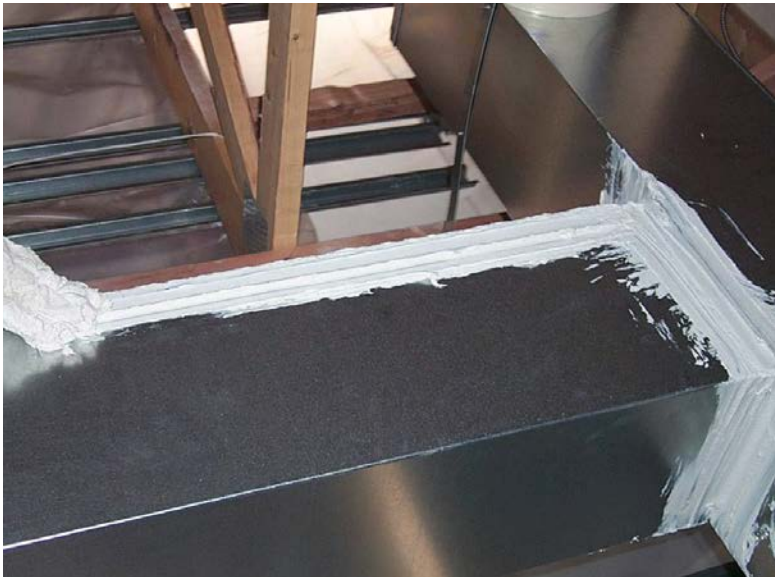
Metal Ductwork Sealed with Mastic ( Click to Return to Section )
